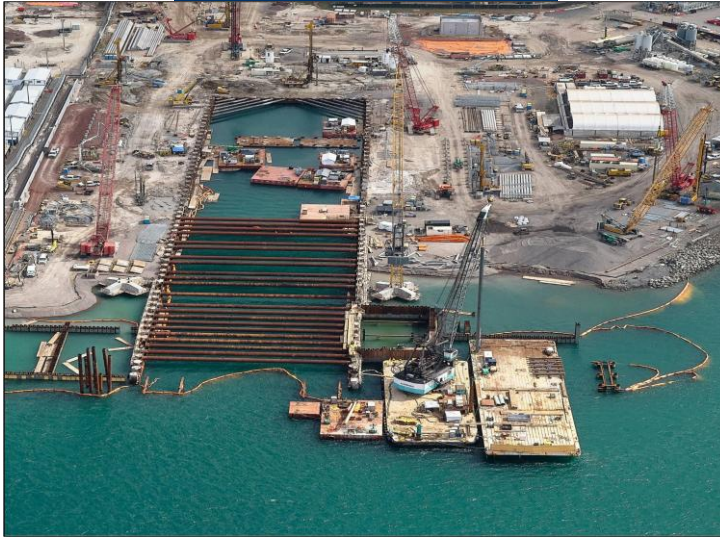
PHNS Dry Dock 5
